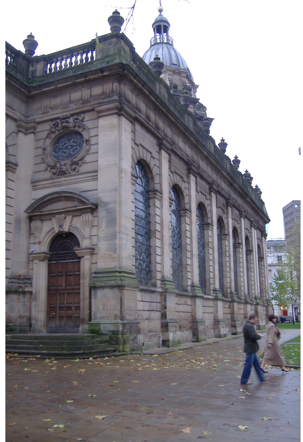
St Philip's – North aisle elevation. Rusticated arches set within pilasters supporting heavy entablature.
