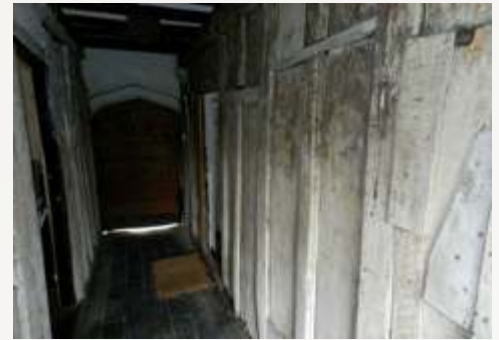
Interior view showing the cross-passage which runs the full depth of the building between the two dwellings; the floor is formed of rectangular blue setts of 19 th century origin and accessed by two stone steps up from the street level
