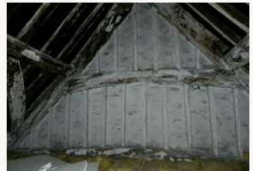
Roof structure and central dividing screen visible within the roof space above No. 6 Thomas Street; note curved wind brace between purlins (lower purlin obscured by (raised) ceiling structure
